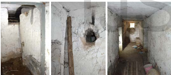
Fig. 10. Openings for ventilation / ventilation of shelters
